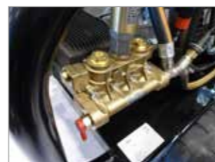
THERMOSTATIC VALVE PROTECTING THE PUMP FROM POSSIBLE OVERHEATING
