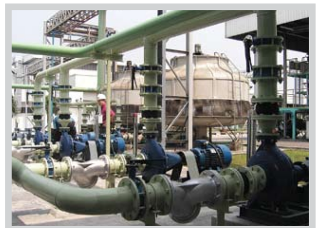
Process Cooling circulation run by EUROFLO centrifugal pump in a car manufacturing plant.
